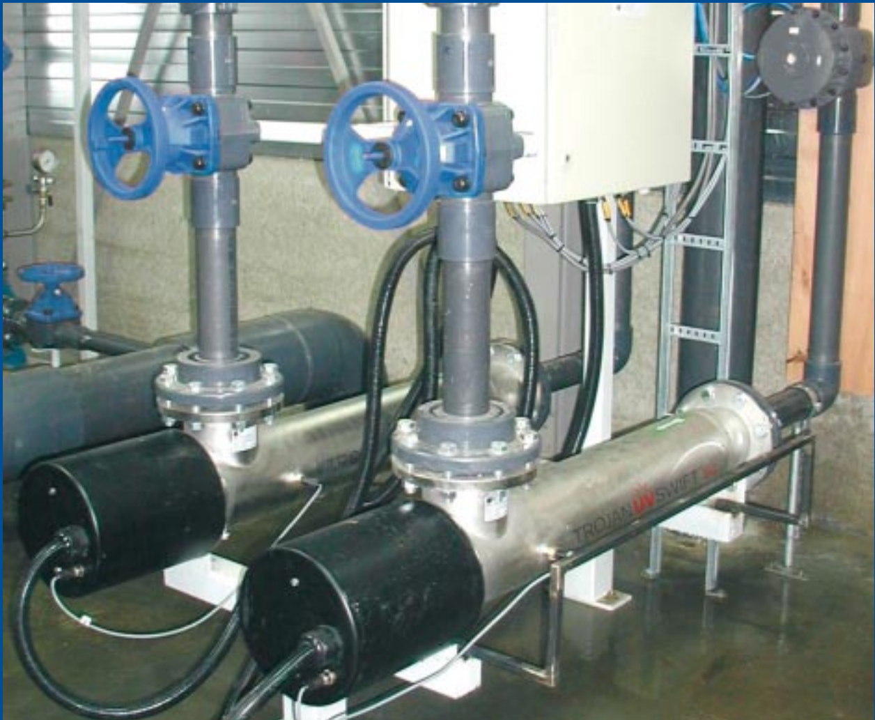
Two Trojan UVSwift™SC units installed in parallel.
